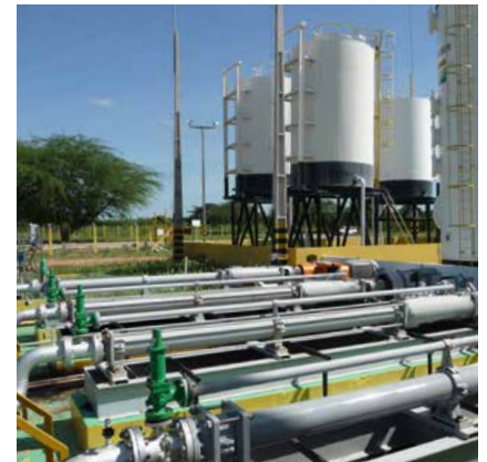
Oil loading pump in Brazil
