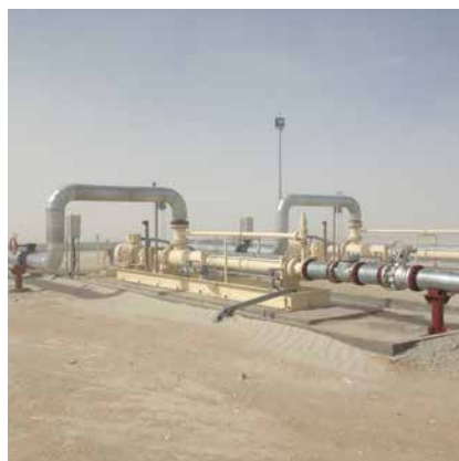
Multiphase pump in Kazakhstan
